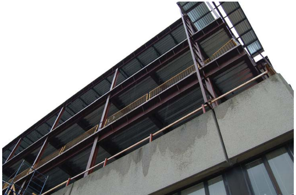
Construction continues at the Burr Wing on the new Cancer Center, mental health unit and more.
